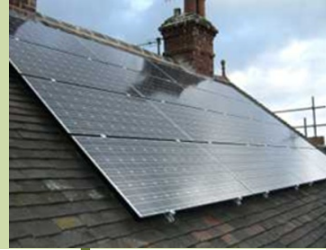
Photovoltaic and solar panels
