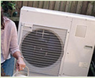
Air source heat pumps
