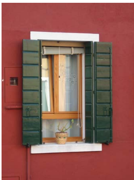
Figure D. An example of external shutters used in the Mediterranean region.
